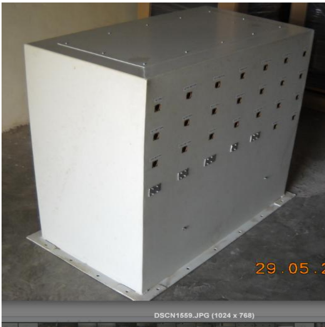
Figure26: Image of cable duct mounted on shielded room
